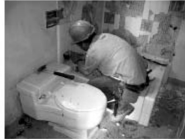
A TRP crew member carefully removes antique decorator tiles from the around the bathtub. They were later incorporated in Jesse Cool's new bathroom.
